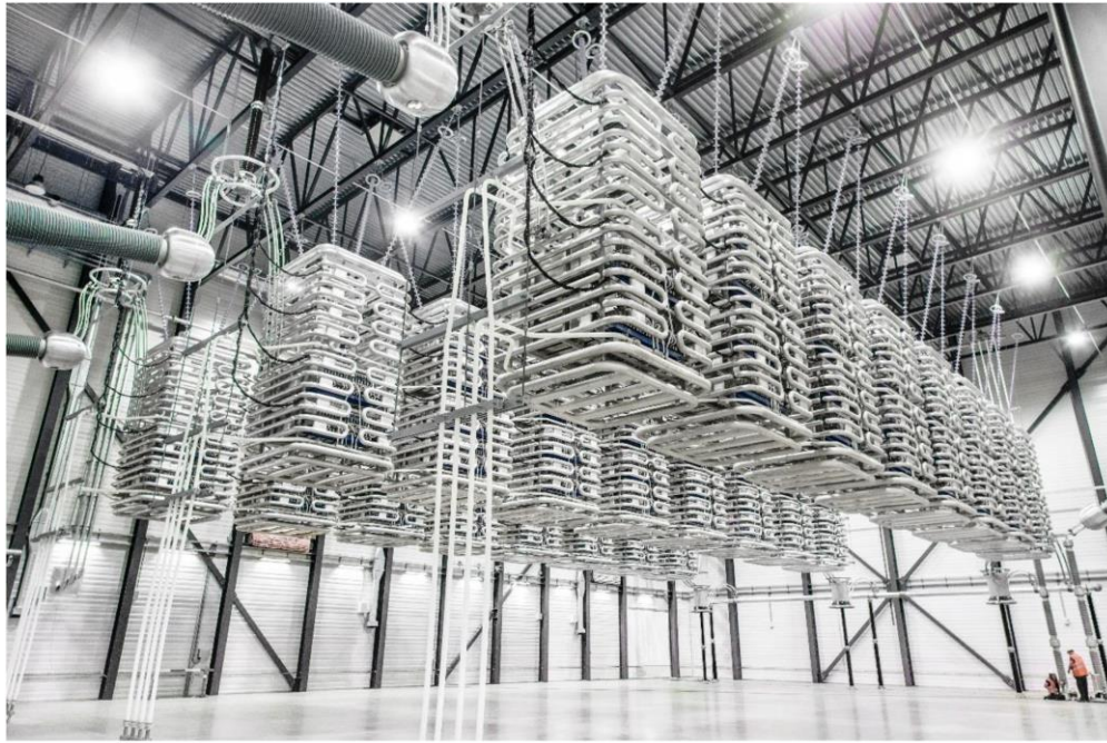
Converter \pm 320 kV/ 700 MW, technology ABB called HVDC Light , Station Skaggerak 4
