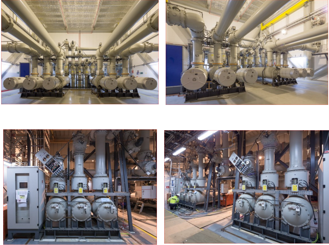
Fig. 11. View of GIS 400 kV type ELK-3 installed on the DolWin-2 platform : HVDC Converter Station with a power value of 924 MW , protected autotransformer and converter devices against short circuit current , generated in large Wind Farm Complex.
